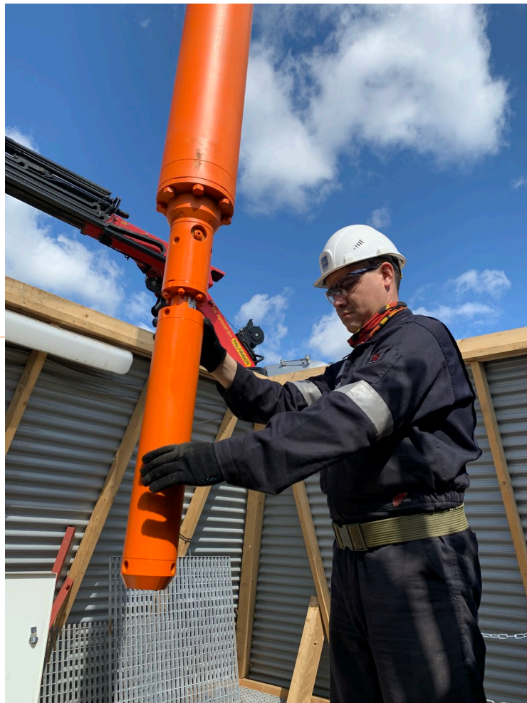
This Geyser GSP system doubled production compared to the previous line-shaft pump and reduced power consumption by 25–30% compared to other geothermal submersible pumps
